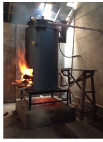
Fire Wood Boiler
