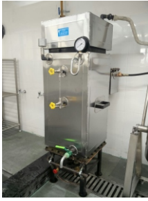
Steam Boiler L.P.G Operated
