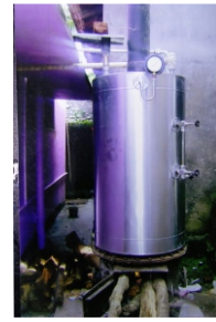
Fire Wood Boiler With Cladding
