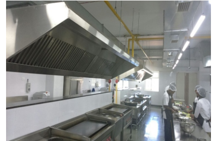
Kichnen Setup With Exhaust System
