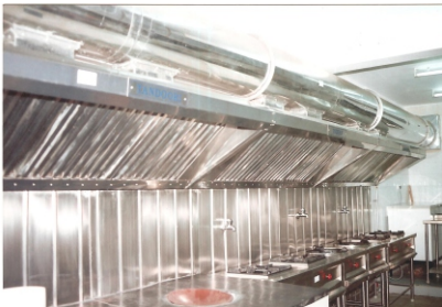
St. Steel Wall Glazing with Exhaust System
